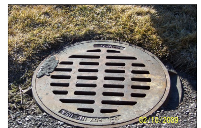
Storm drain producing mosquitoes.
