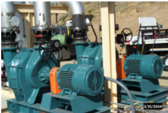
Figure 9 Motors and Compressors
