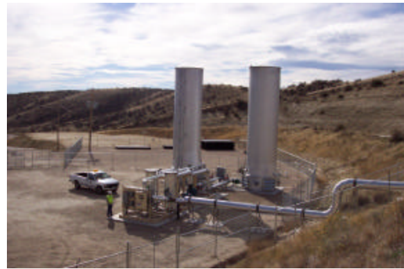
Figure 10 LF Gas Flare Station
