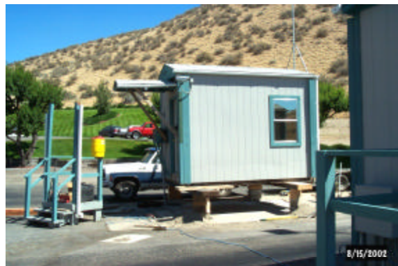
Figure 16 - Cashier's Booth on stilts awaiting new support.
