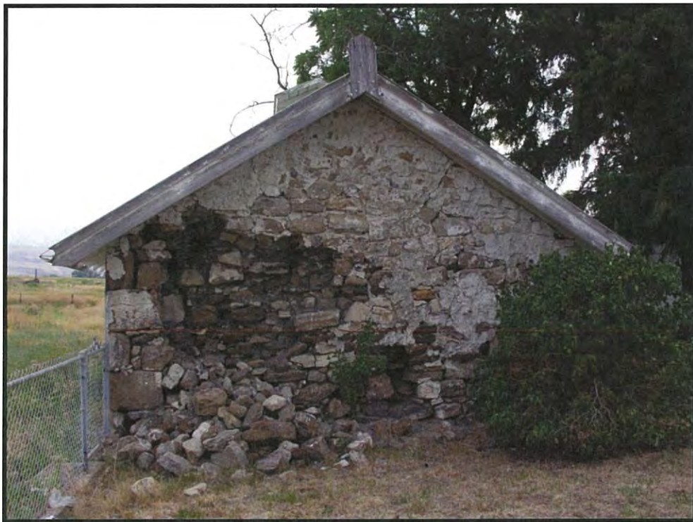
Figure 30 Feature 5, Cold House, to the damage to west wall (DSCN4239; 06/18/2016).
