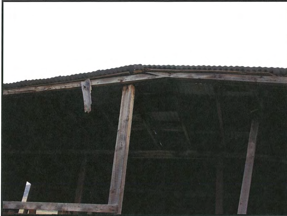
Figure 13. Feature 1 Dairy Barn detail showing damage (DSCN4197; 06/18/2016).
