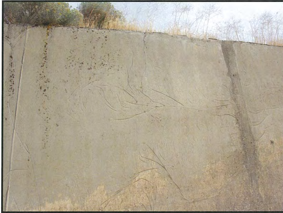
Figure 53. Feature 12, Silage Pit, detail of concrete walls showing imprint of plastic sheets used to protect the forms (DSCN4183; 06/18/2016).
