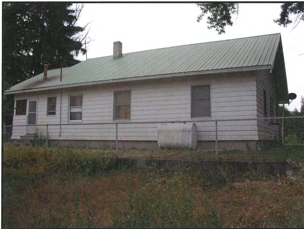
Figure 26. Feature 4, Dwelling, to the south, southeast (DSCN4228; 06/18/2016). Note concrete retaining wall protecting the north side of the structure.
