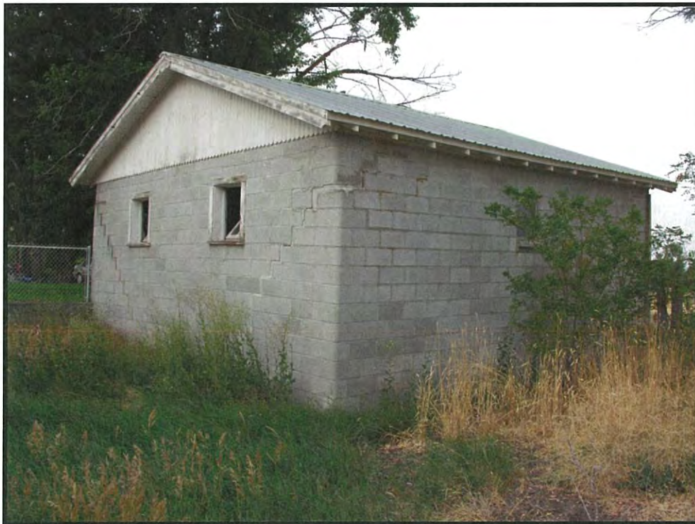
Figure 22. Feature 3, Cinderblock Garage, to the northeast (DSCN4219; 06/18/2016). Note damage to the corners of the garage from slumping foundation
